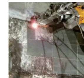
Anti-cavitation coating on hydro power station
